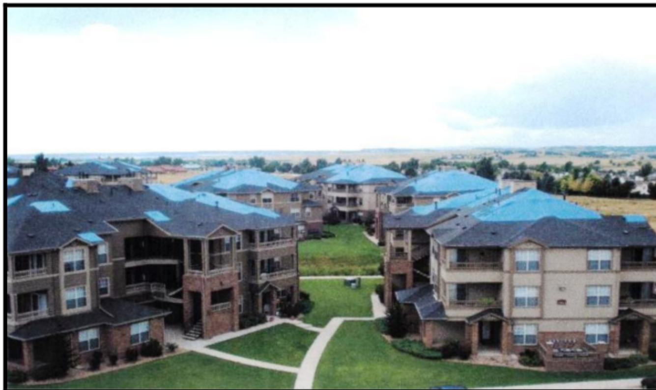
Figure 2 Photo shows numerous small and large tarps carefully applied to damaged roofs 3 story structures
