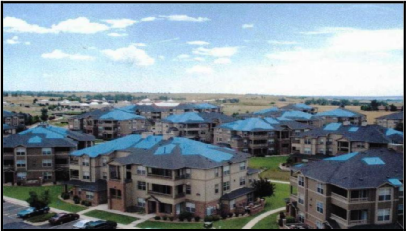
Figure 3 Photo shows numerous small and large tarps carefully applied to damaged roofs 3 story structures
